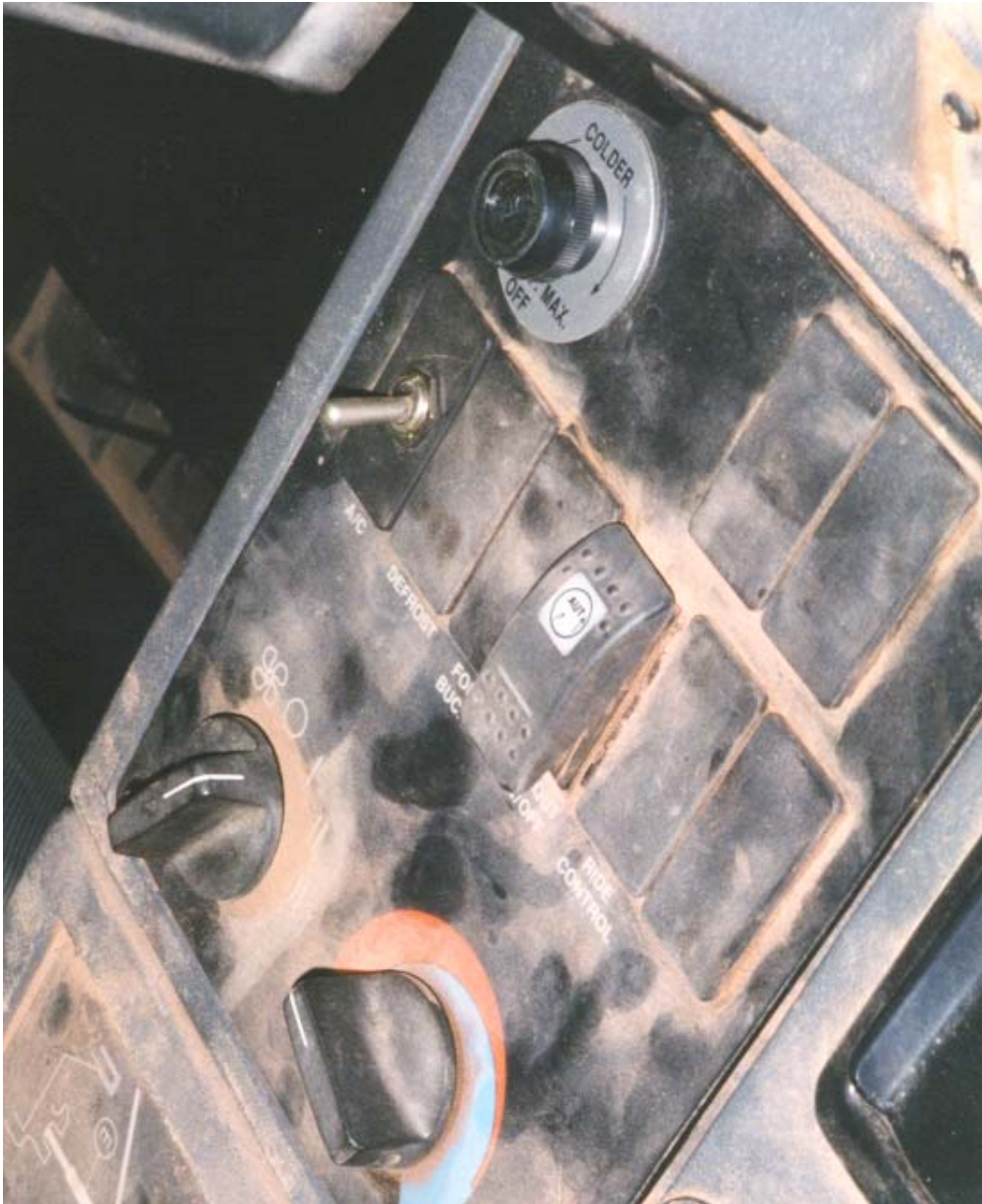
Thermostat in place on control panel.
