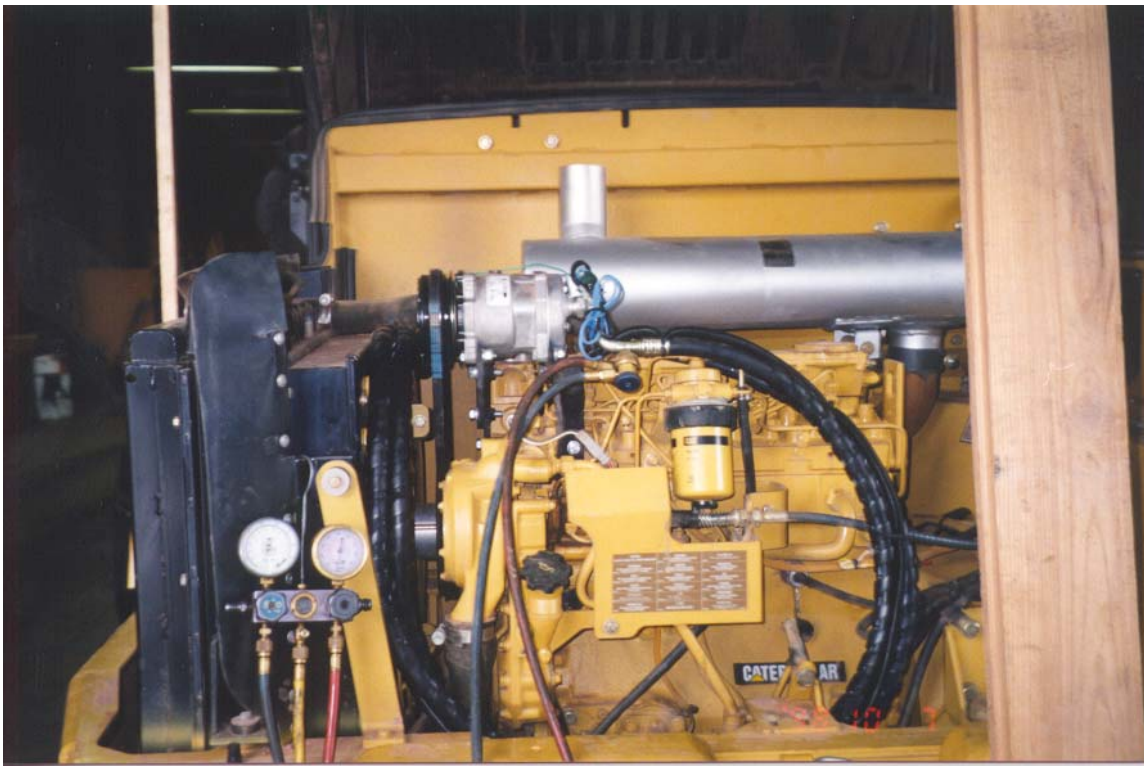
Compressor in place showing line runs.
